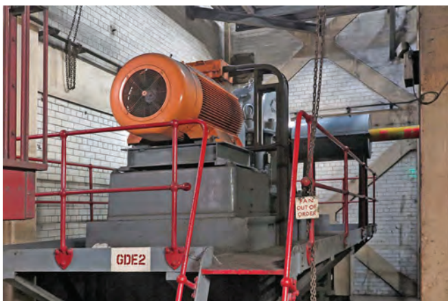
The 1930s engine to run the huge fans that pull foul air and fumes from the ceiling of the tunnel, to be vented through the high chimney of the building. Photo Clive Penfold
